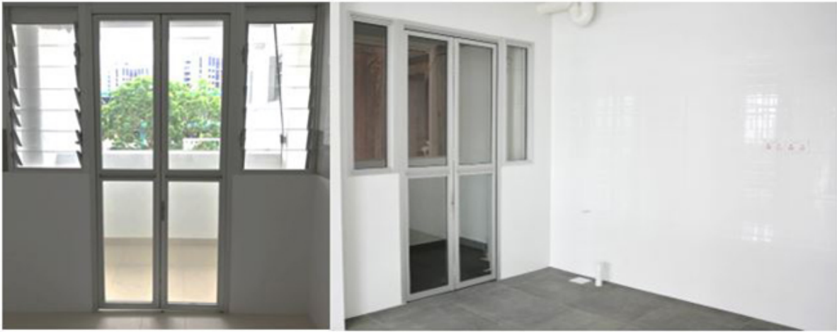
The louvered windows in the door/window ensemble between the kitchen and service yard (left) will be replaced with top-hung windows (right), allowing for more flexibility in the layout of kitchen furniture.
