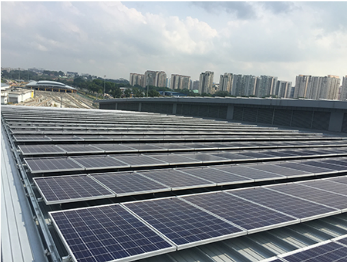
Solar panels at Gali Batu Depot
