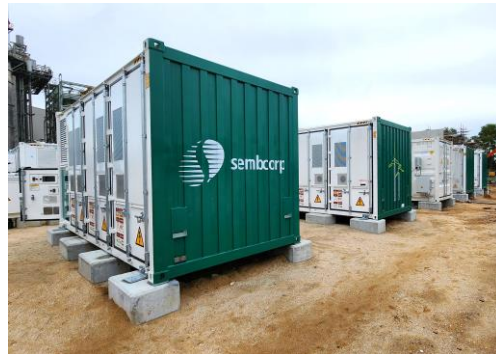
Sembcorp developed a 285MWh ESS, which has been operational since Dec 2022. It is the largest ESS deployment in Southeast Asia, and one of the fastest of its size to be deployed.
