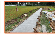
Construction of concrete footpath sections for environmental field monitoring at Temasek Polytechnic
