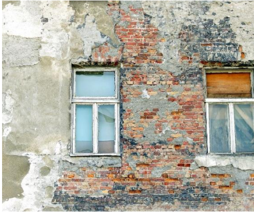
(a) Erosion of building surfaces
