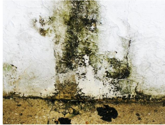
(b) Mold growth on building structures
