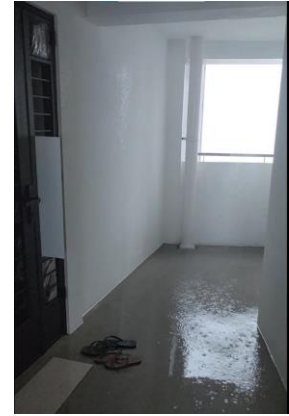
(c) Flooding and slipping hazard
