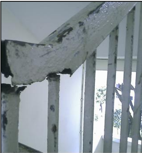
Corroded staircase railings
