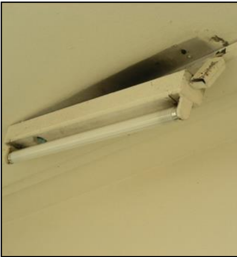
Dangling ceiling light fitting
