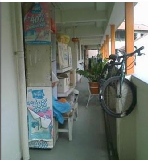
Obstruction of corridor
