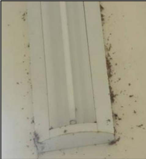
Cobwebs on light fitting
