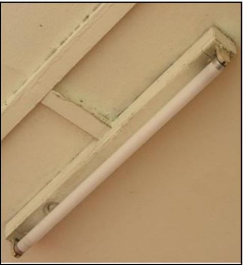
Light fitting firmly affixed to ceiling
