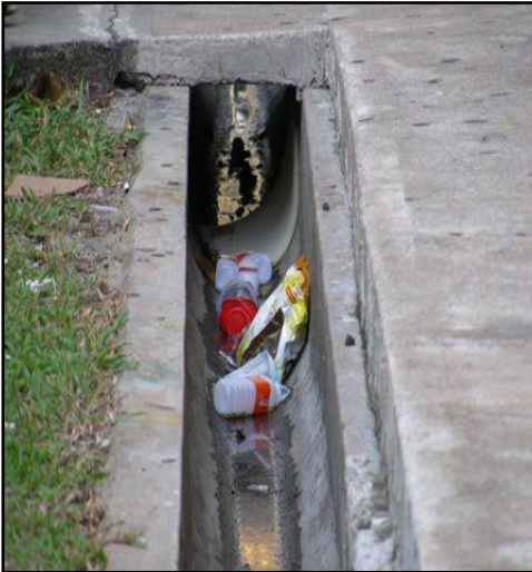
Litters in apron drain
