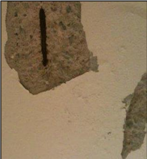
Spalling concrete on corridor ceiling
