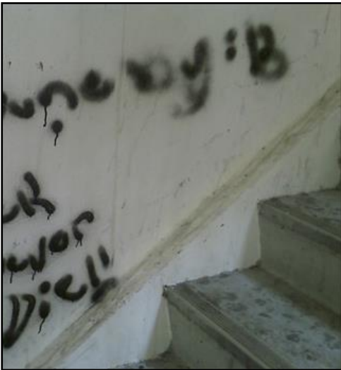
Wall stained with graffiti
