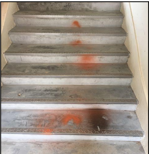
Stain on staircase
