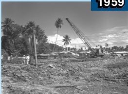
Construction works in Singapore, 1959. Photo credit: Ministry of Information and the Arts Collection, courtesy of National Archives of Singapore
