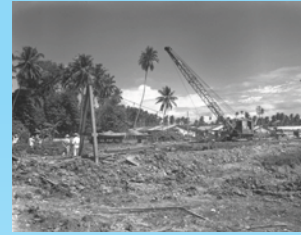
Construction works, 1959 Photo credit: Ministry of Information and the Arts Collection, courtesy of National Archives of Singapore
